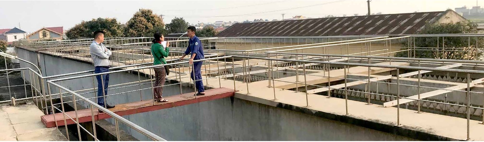
Filtering tank at water plant Giao Thuy, Nam Dinh province.
