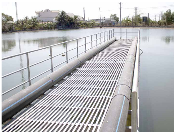
Raw water suction pipe at the central water plant of Ham Thuan Bac district, Binh Thuan province.
