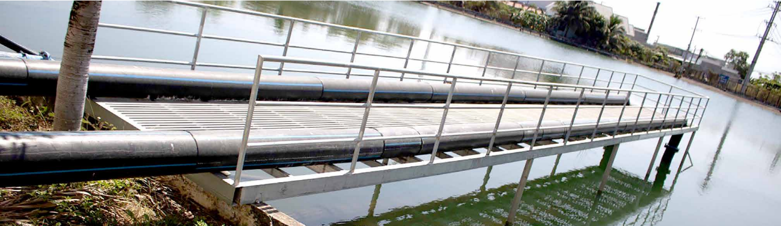
Raw water suction pipe at the central water plant of Ham Thuan Bac district, Binh Thuan province.
