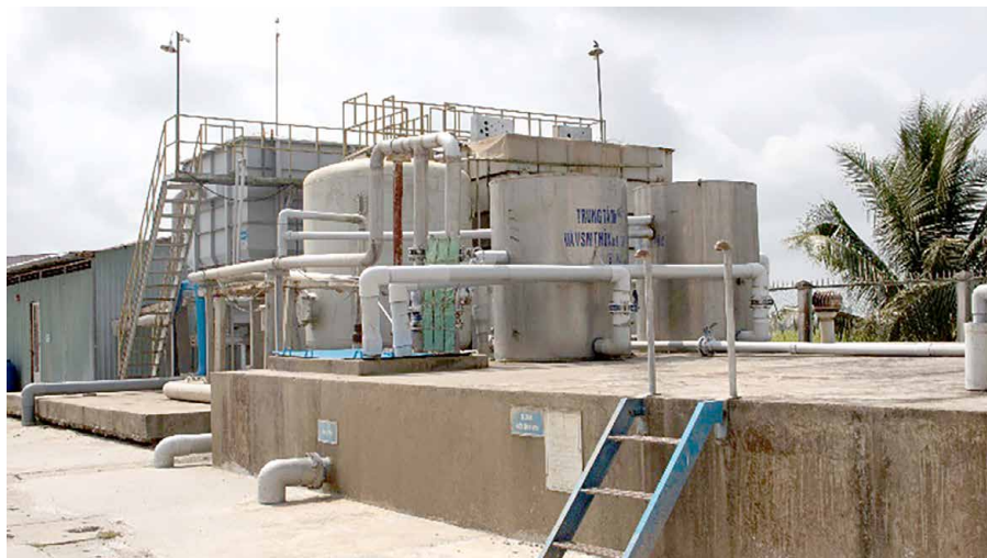
Centralized water supply system in Thanh An, Thanh Thang-Thanh Loi commune, Can Tho province.
