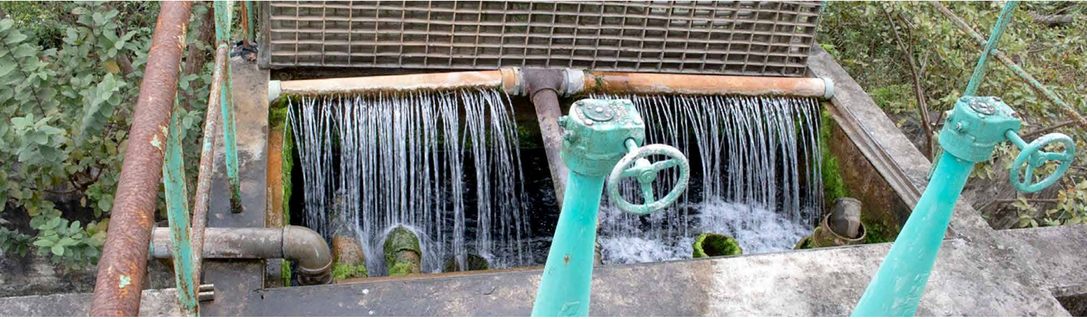
Filtering tank of Hoa Thuong water plant in Thai Nguyen province.
