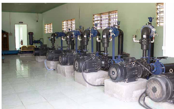
Water pump system at the central water plant of Ham Thuan Bac district, Binh Thuan province.
