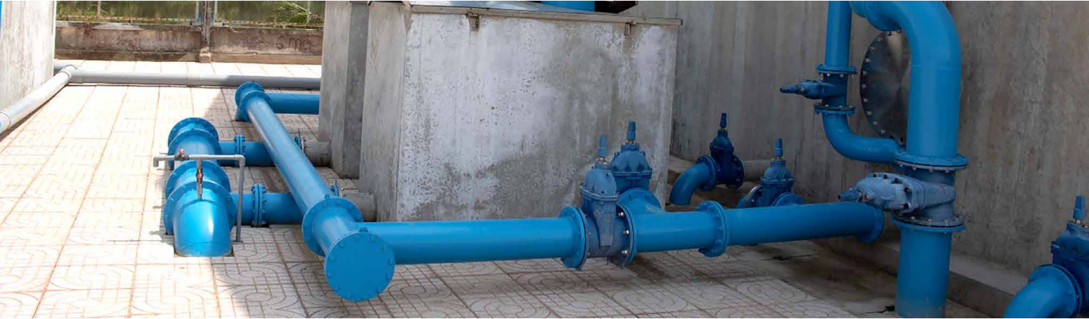
Treatment water pipeline in the centralized water supply system of Thanh An, Thanh Thang-Thanh Loi commune, Can Tho province.
