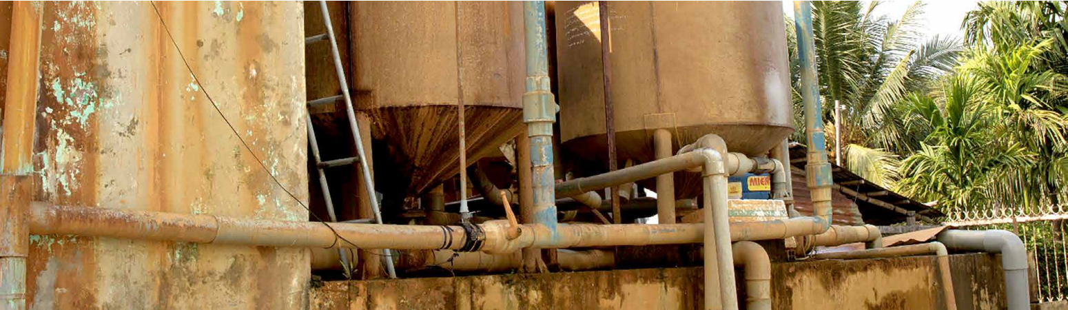
Centralized water supply station in My Huong commune, Soc Trang province.
