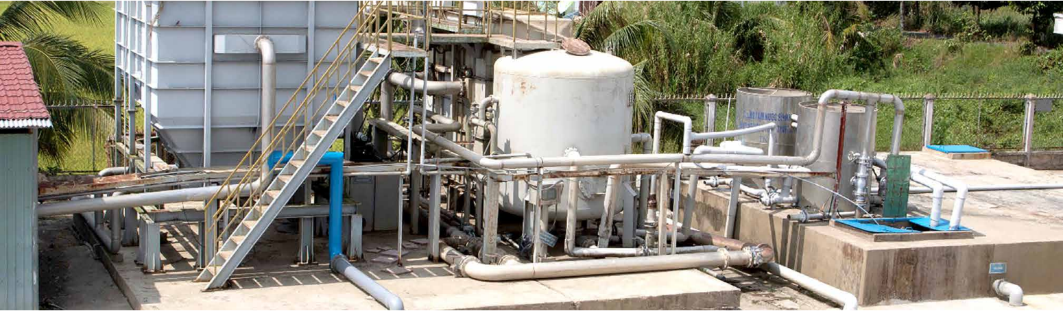
Centralized water supply system in Thanh An, Thanh Thang-Thanh Loi commune, Can Tho province.
