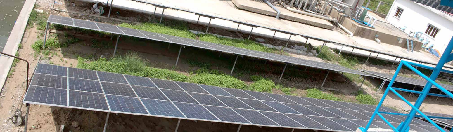
Solar power system installed at the centralized water supply system in Thanh An, Thanh Thang-Thanh Loi commune, Can Tho province.
