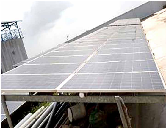
Solar power system in Thanh An, Thanh Thang-Thanh Loi commune, Can Tho province.
